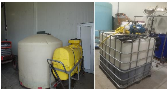
Diluted Tanks for Spraying
